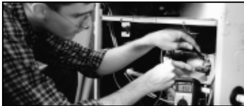
Poorly functioning motors may just be the result of a bad capacitor.
